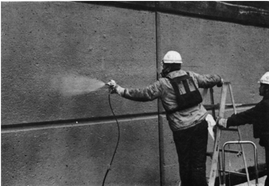
Spraying lock wall with icephobic coating developed by CRREL, Sault Ste. Marie, Michigan.
